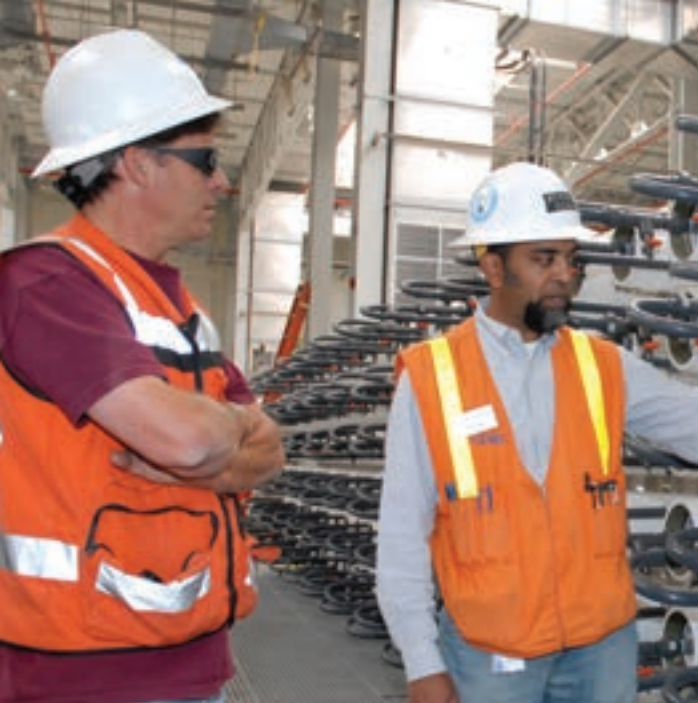
Orange County Water District Principal Engineer and GWRs Program Manager Mehul Patel (right) examines reverse osmosis connections in the District's Groundwater Replenishment System (GWRs). The system provides a high-quality source of water to recharge the county's groundwater basin.
